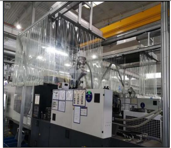
注塑废气集气罩+软帘
